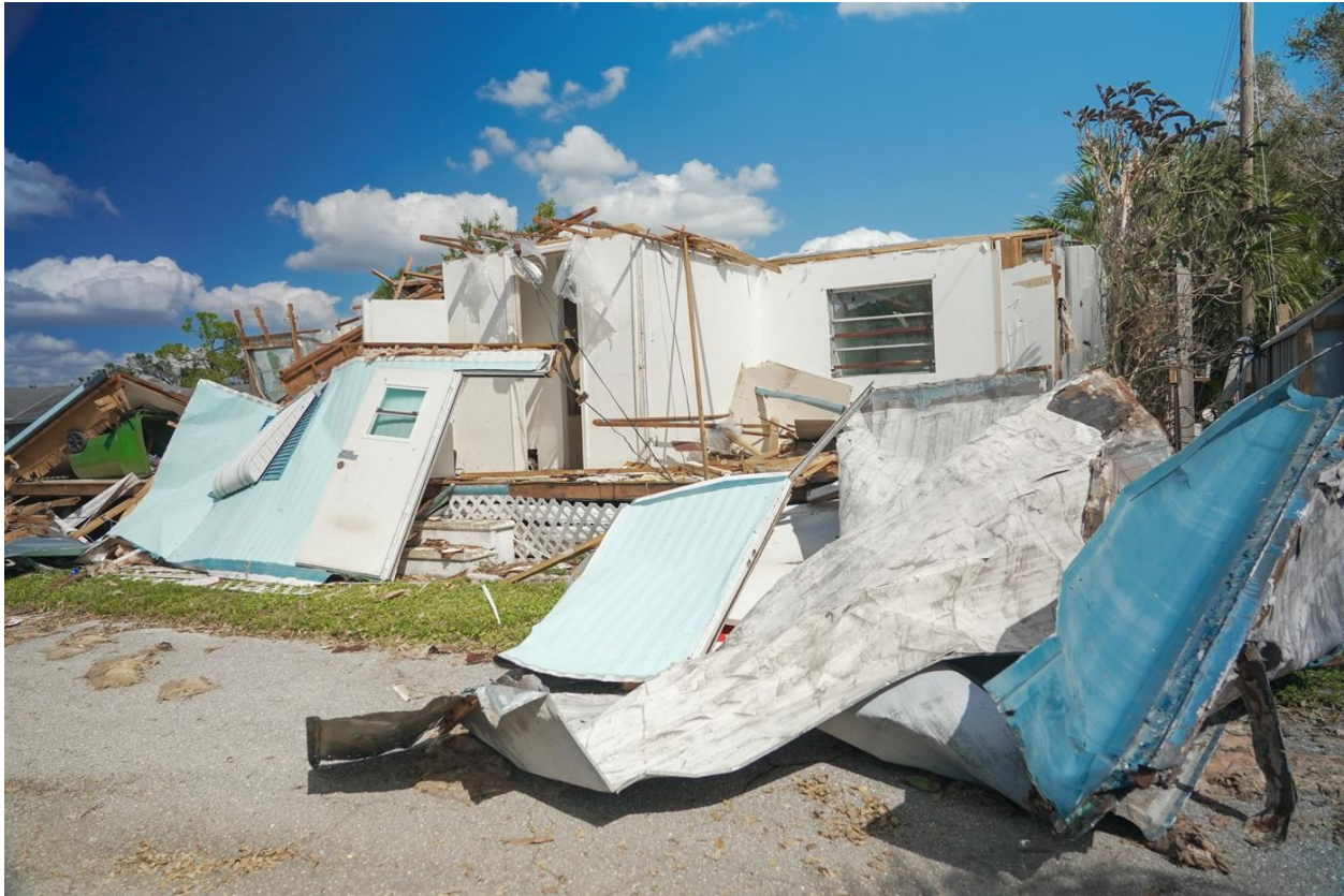
Figure 11 – Hurricane Milton Modular Home Damage
